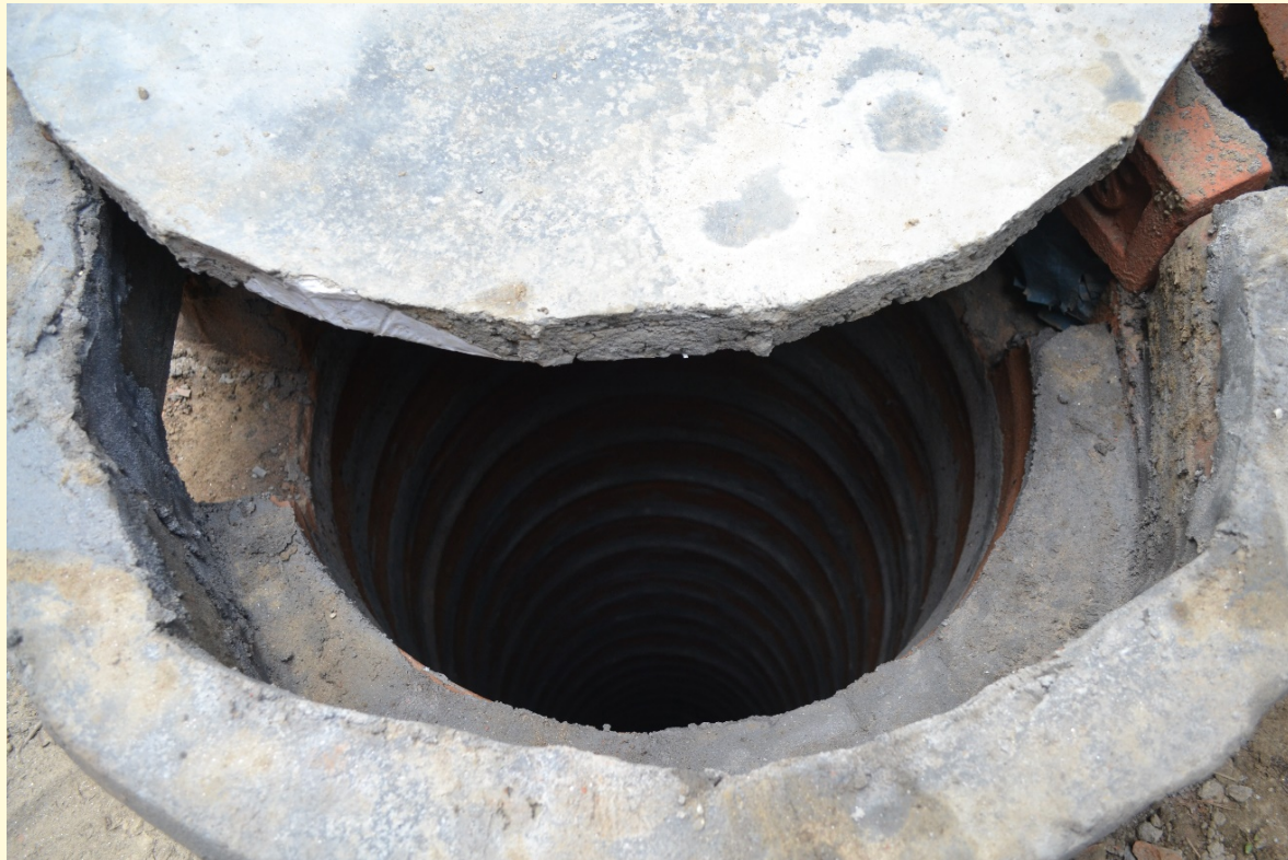
Vertical distance between ground water level and soak pit not maintained
