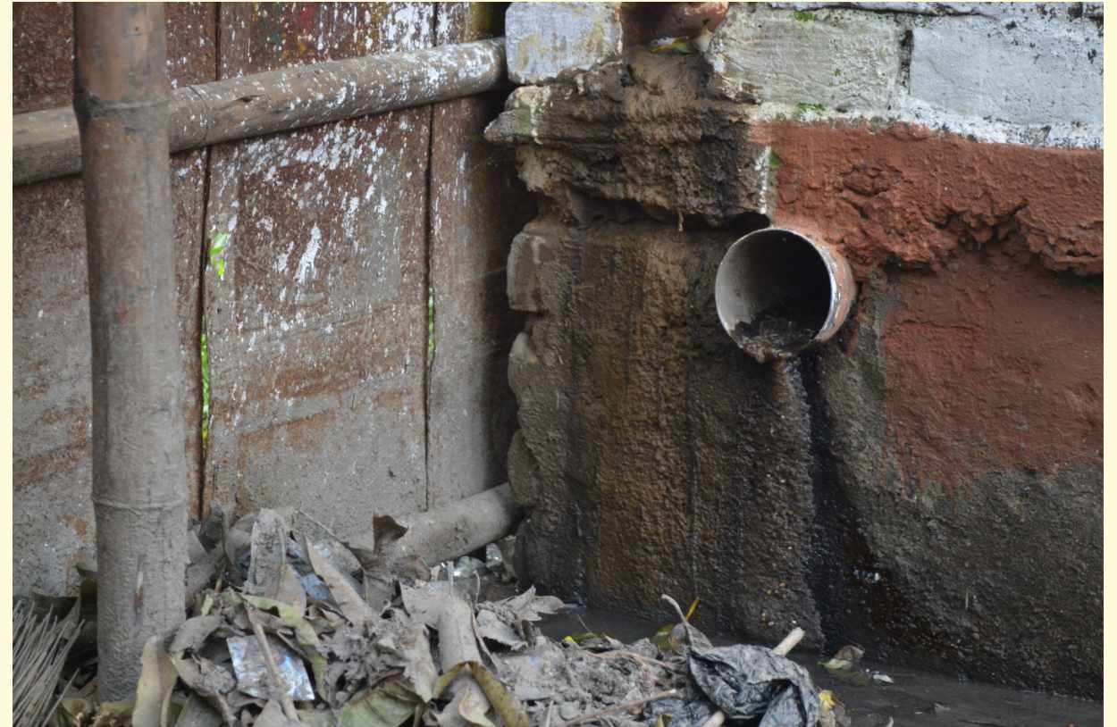
Effluent let off in the open drains
